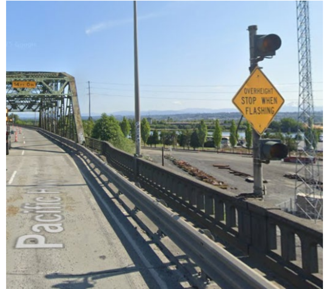
WSDOT advance warning system at northbound SR 529 over the Snohomish River near Everett
