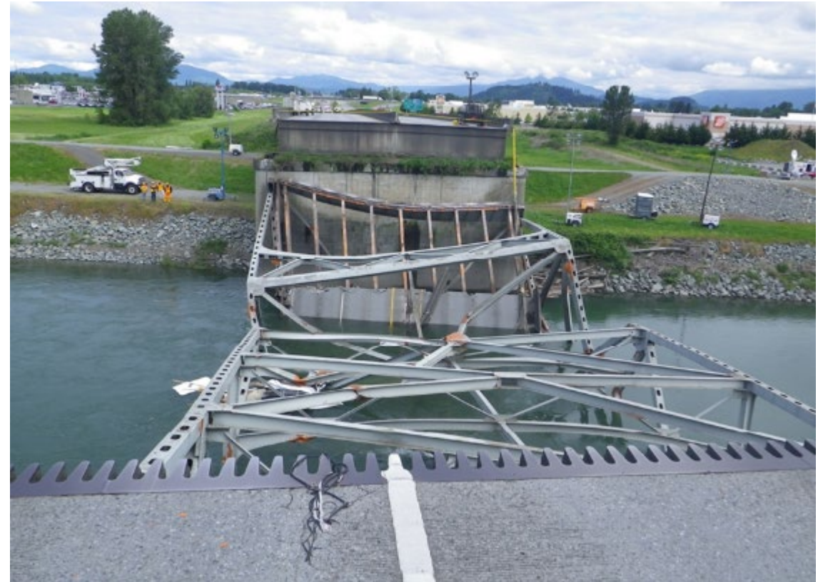
2013 Collapse of the I-5 Bridge span over the Skagit River
