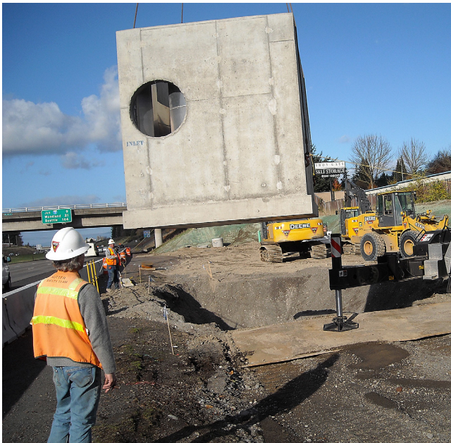
Stormwater retrofits — like this one being installed in Vancouver, WA — reduce pollution in stormwater runoff and protect coho salmon and other aquatic wildlife.
