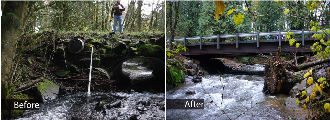
Fish passage projects like this one on Baxter Creek in Cowlitz County replace culverts and restores access to valuable habitat for salmon. (Photos: Washington State Recreation and Conservation Office)
