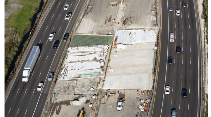
SR 167 Stage 1b: When inner bridge lanes are complete, traffic will shift towards the I-5 median while crews work on outer bridge portions in Fife.
