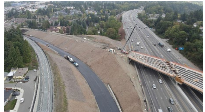
SR 509 Stage 1b: Crews set girders for the new bridge over I-5 and continue work to complete the bridge deck.
