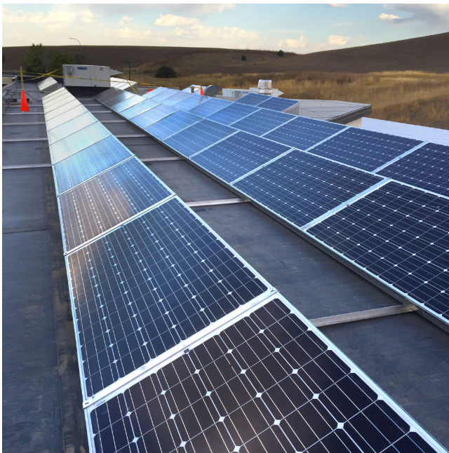
Roof array of solar panels on a Washington State University building. The governor is proposing investments to make state agency facilities more energy efficient, including solar installations.
