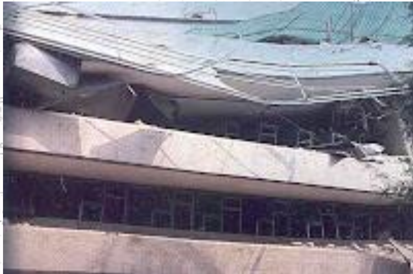
School building collapse in Mexico earthquake 1985. Photo credit unknown
