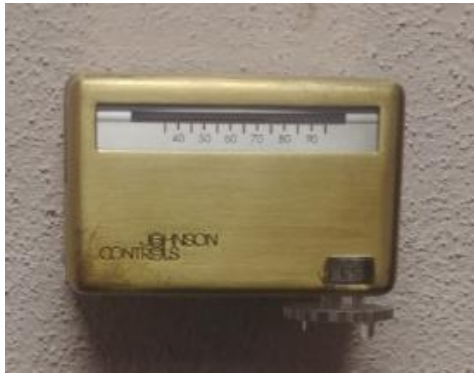
Pneumatic Thermostat (Installed in 1987)
