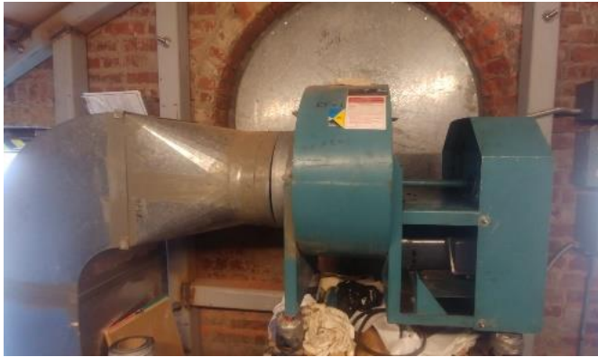
Exhaust Fan in Attic Space
