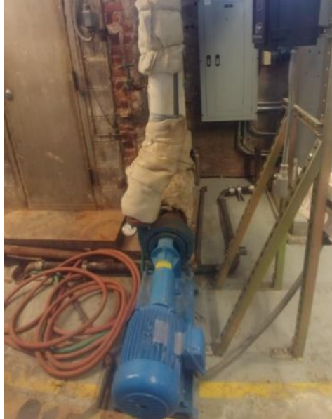
Chilled Water Pump
