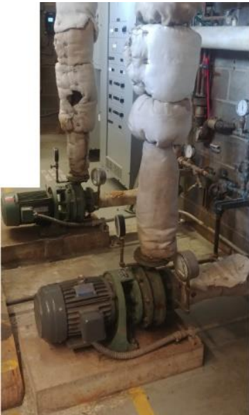
Heating Water Pumps
