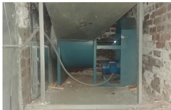
Smoke Evacuation fans (SF-3 and SF-4)
