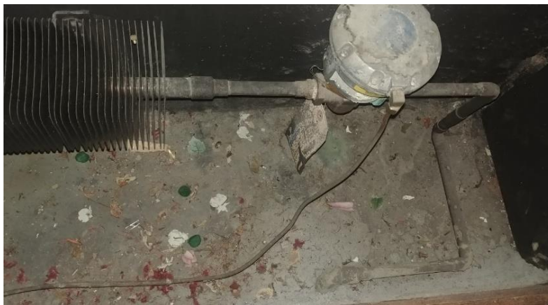
Radiator and Pneumatic Control Valve. Shows HW piping buried in concrete
