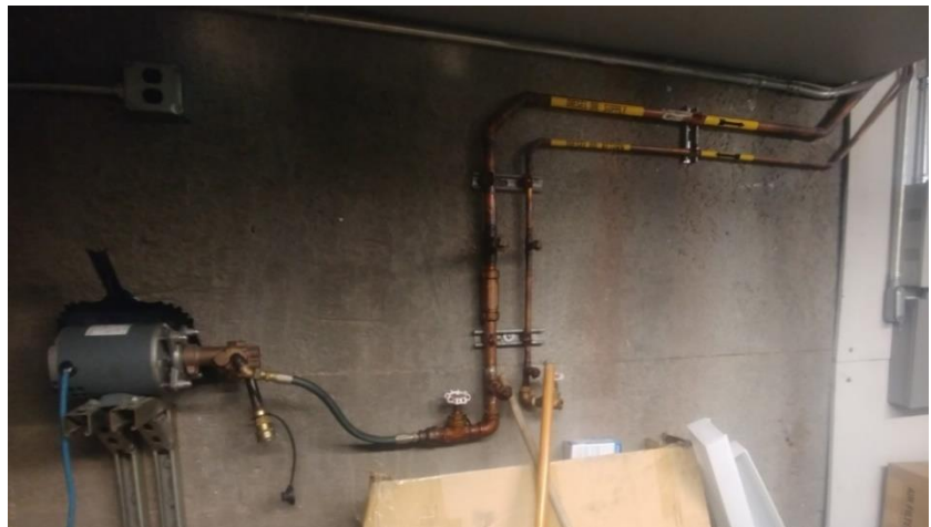
Diesel Generator on Roof and fill piping in lower mechanical room
