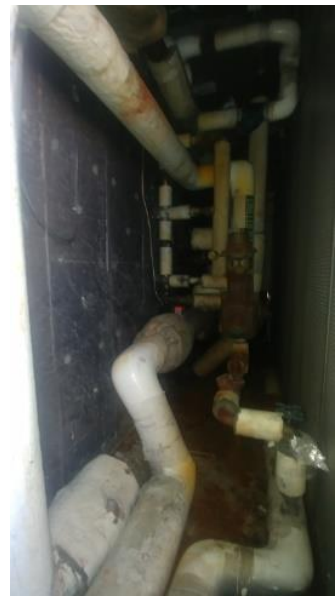
Steam and CHW piping
