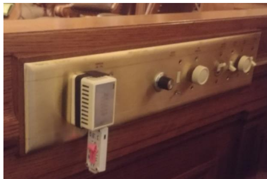
Dimming Panel in Courtroom
