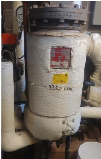
Steam to Hot Water Heat Exchanger
