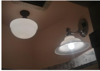
Typical Restroom Type Fixtures
