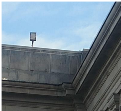
Exterior Lighting – LED
