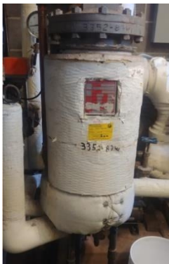
Steam to Hot Water Heat Exchanger
