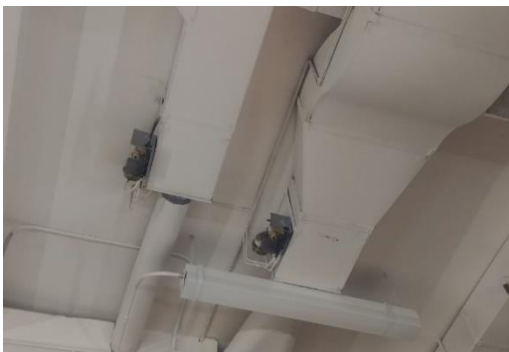
VAV Boxes (box with a pneumatic damper)
