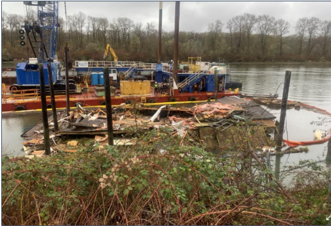
Figure 4. Float house structure collapsed in on itself, 04/10/2023.
