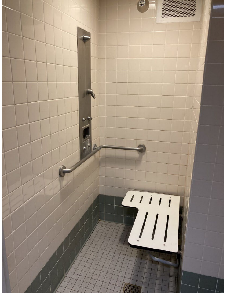
Image 25: ADA solitary confinement shower at Washington Corrections Center for Women (WCCW).
