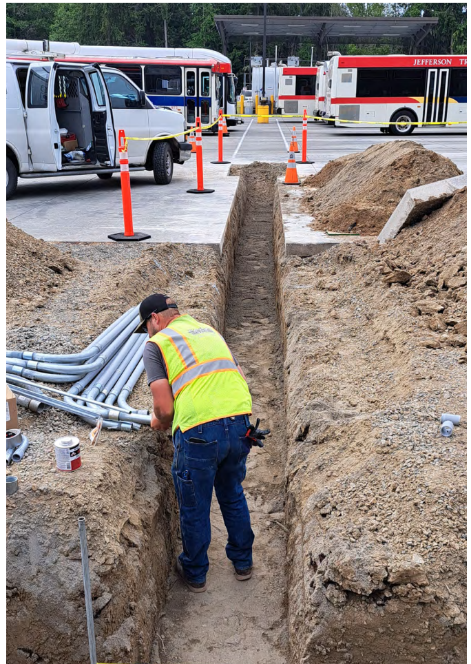
A worker digs a trench for EV charging infrastructure at a Jefferson Transit Authority station in Jefferson County.
