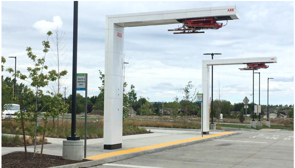
High-powered electric bus chargers shown at a bus depot.
