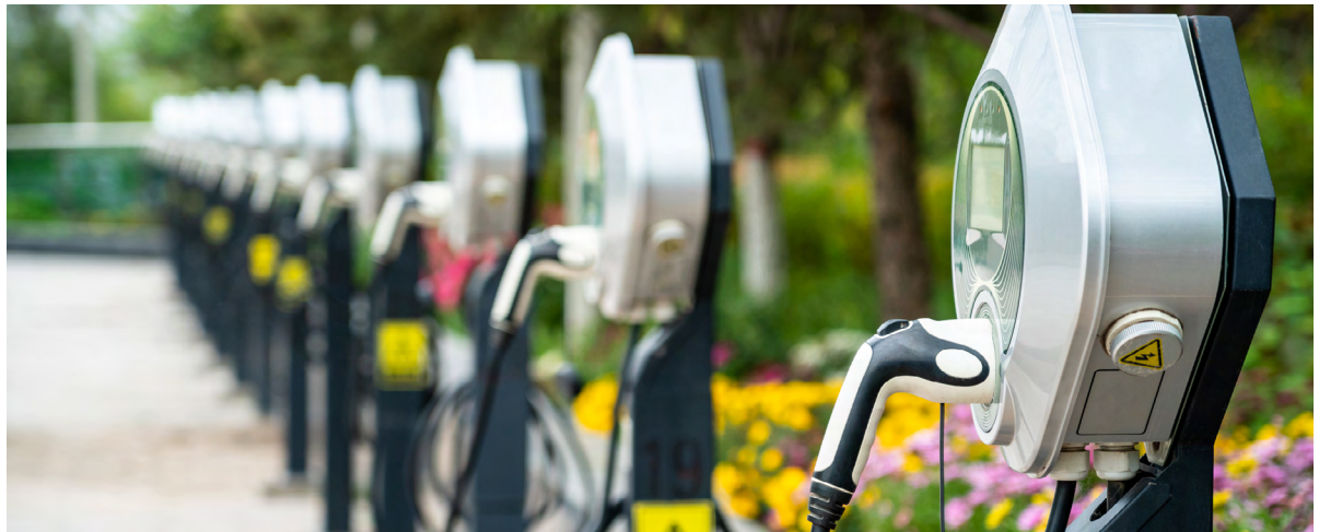
A row of electric vehicle chargers ready for use.
