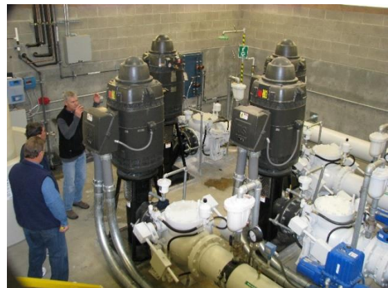
City of Kennewick wastewater treatment facility Seeing how it all works.
