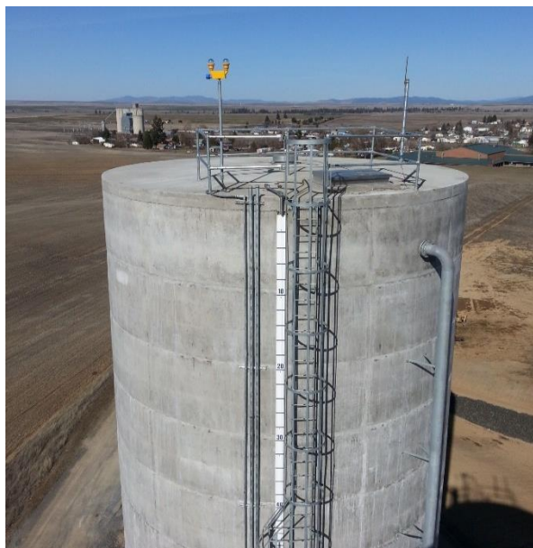
Town of Creston Water reservoir.
