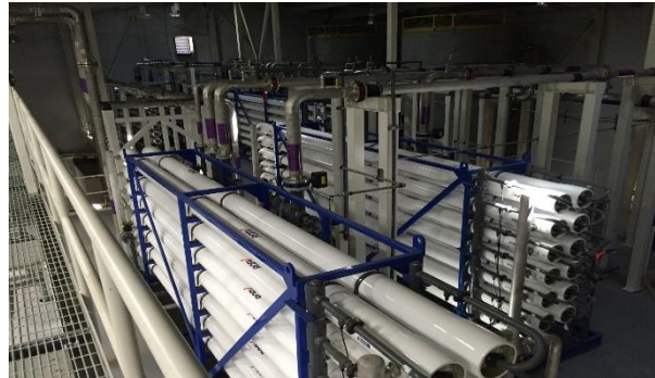
City of Quincy reverse osmosis membrane Project co-funded by state and federal agencies.
