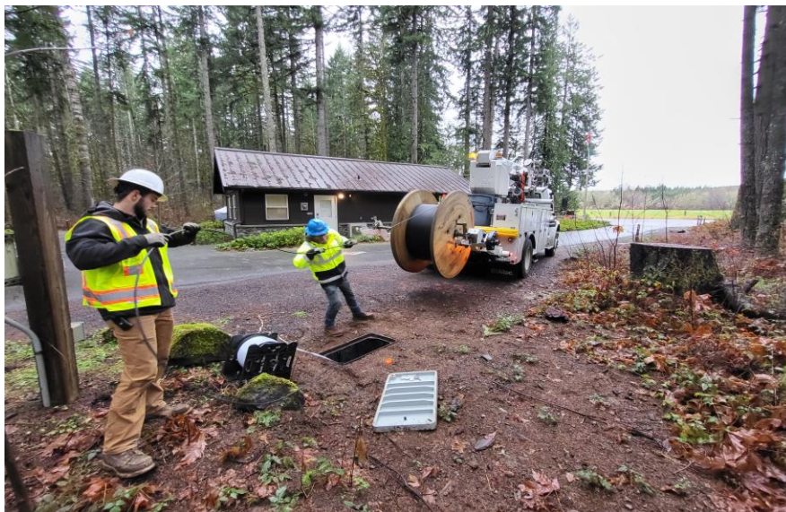
Lewis County Public Utility District preparing to install fiber at Rainbow Falls State Park, December 2023
