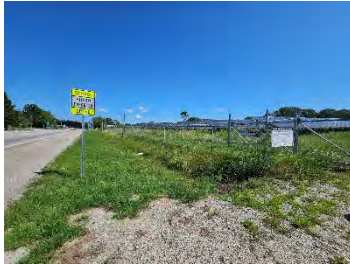
Figure 15: A one-megawatt solar array in the ROW at Exit 14 on I-85 leveraging 2,600 high-efficiency solar panels, with native, pollinator-friendly wildflowers planted under and around the solar panels.
