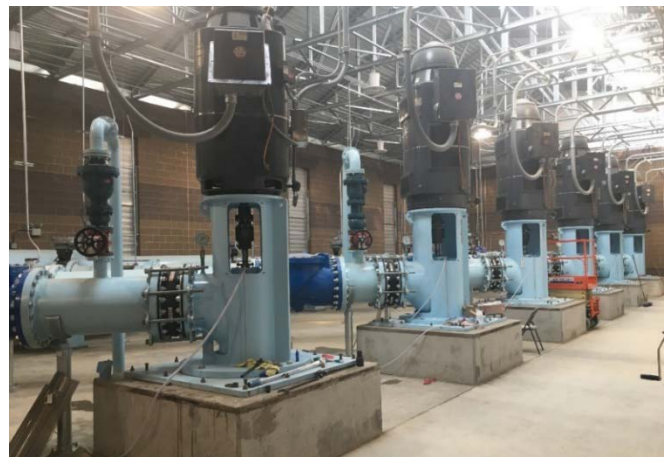
Pumps inside the EL 47.5 Pumping Plant
