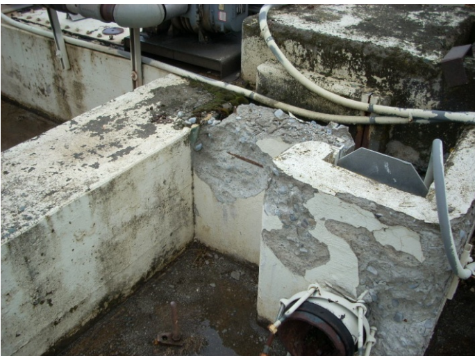
Part of the aging Tekoa wastewater treatment plant. Flaking concrete and exposed rebar are seen in the center of the photo. Ecology Photo
