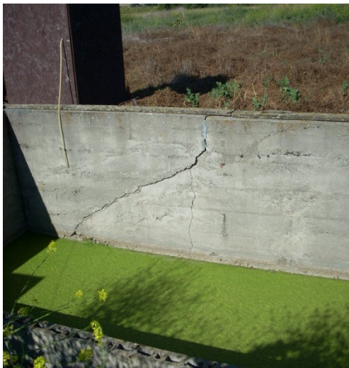
The 45-year old system is showing significant deterioration, as can be seen in the crack in the contact tank used for disinfection. Ecology photo
