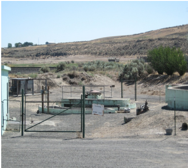
The 55 year old Lind wastewater treatment plant still in operation. Ecology Photo
