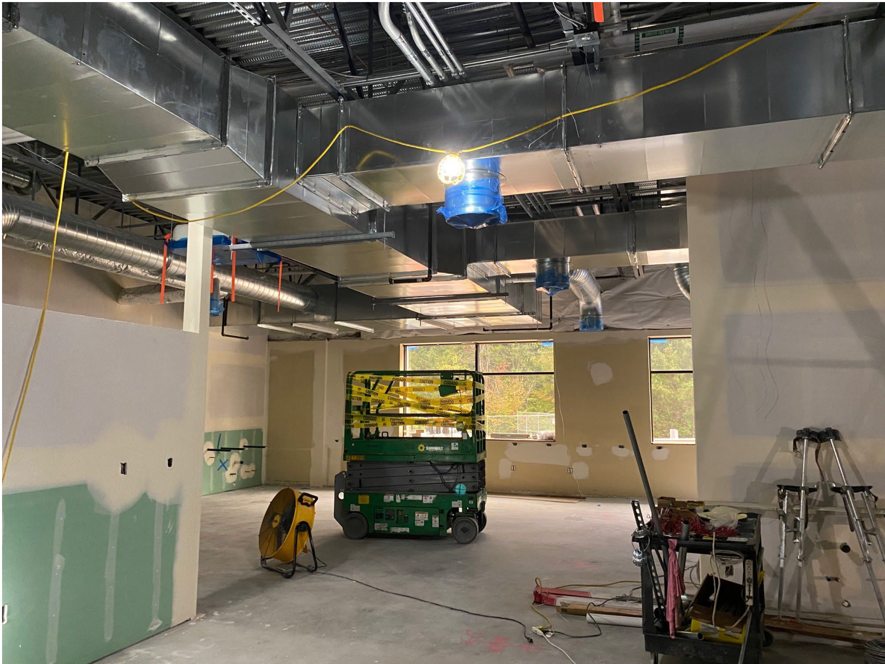
Federal Way Tox Lab – West End of Extraction Lab
