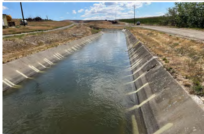
Roza main canal sealing complete. Dry (top) and full (bottom) canal comparison.
