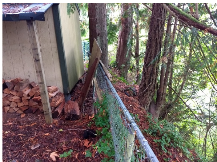
Figure 8. Shed at the Firepit, Very Close to the Edge of an Undermined Bluff.
