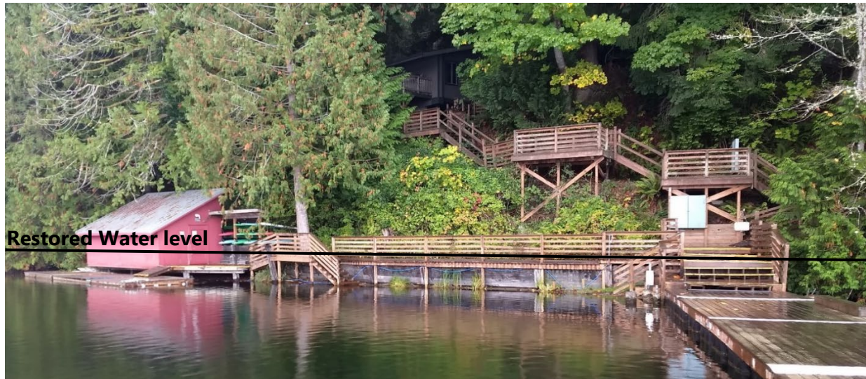
Figure 5. Gangway, Decking, and Access Stairs Will Need to be Rebuilt to Accommodate Restored Water Level.
