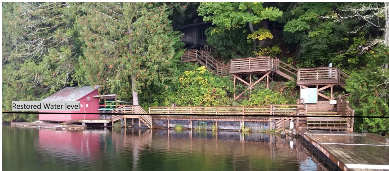
Figure 12. Gangway, Decking, and Access Stairs Will Need To Be Rebuilt to Accommodate Restored Water Level.
