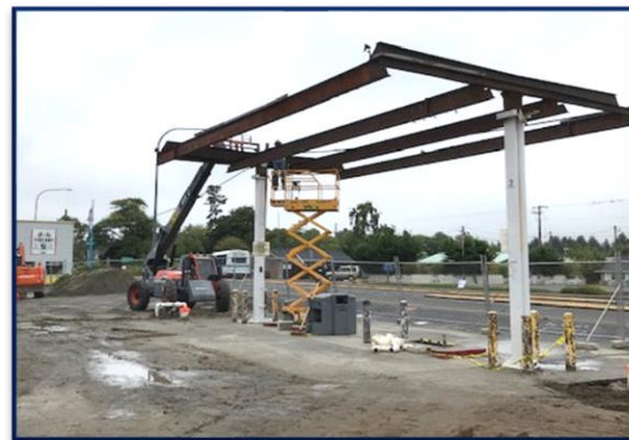
Cleanup and construction included removal of the canopy and dispensers to access tanks.
