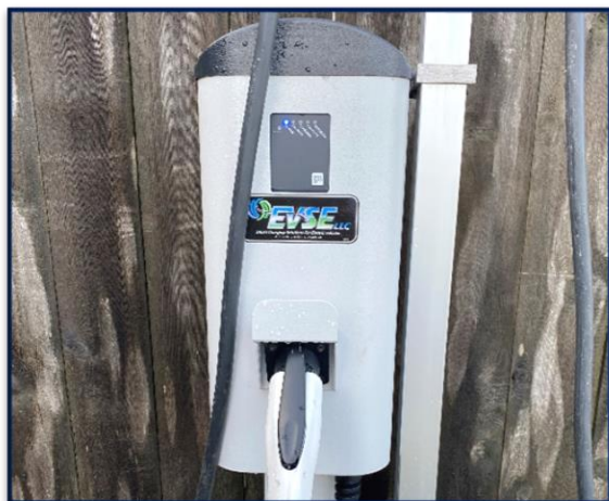
New electric vehicle charging station installed.
